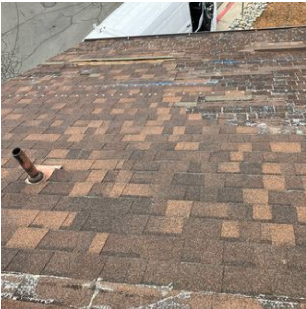
File Name:Ricardo pics_0018.jpg Description:Overview pics of damage roof HiRes Image URL: Click Me
