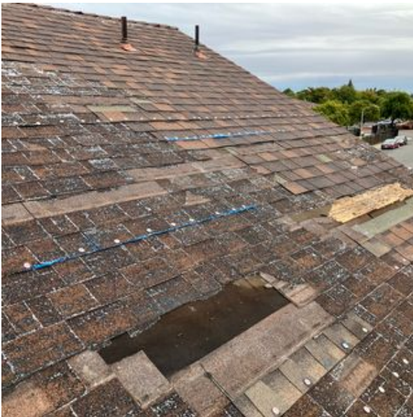
File Name:Ricardo pics_0012.jpg Description:Roof damage HiRes Image URL: Click Me
