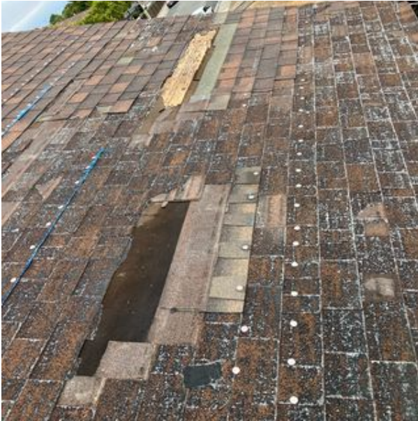
File Name:Ricardo pics_0014.jpg Description:Roof damage HiRes Image URL: Click Me
